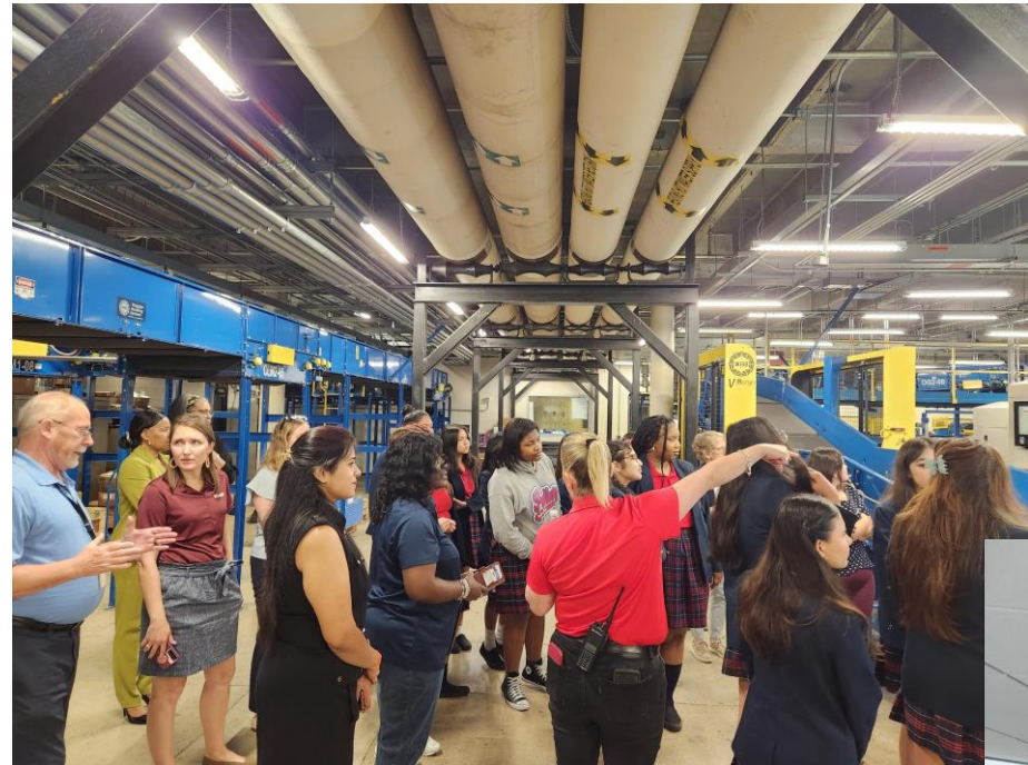
Baggage Handling System
